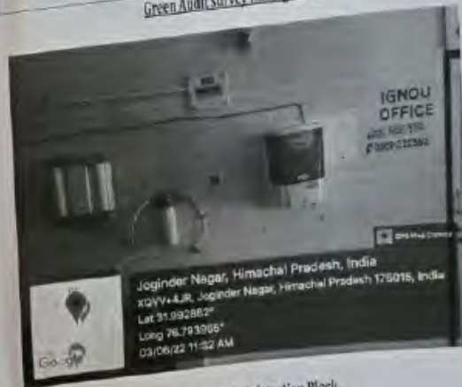
Water purifier in Administration Block
